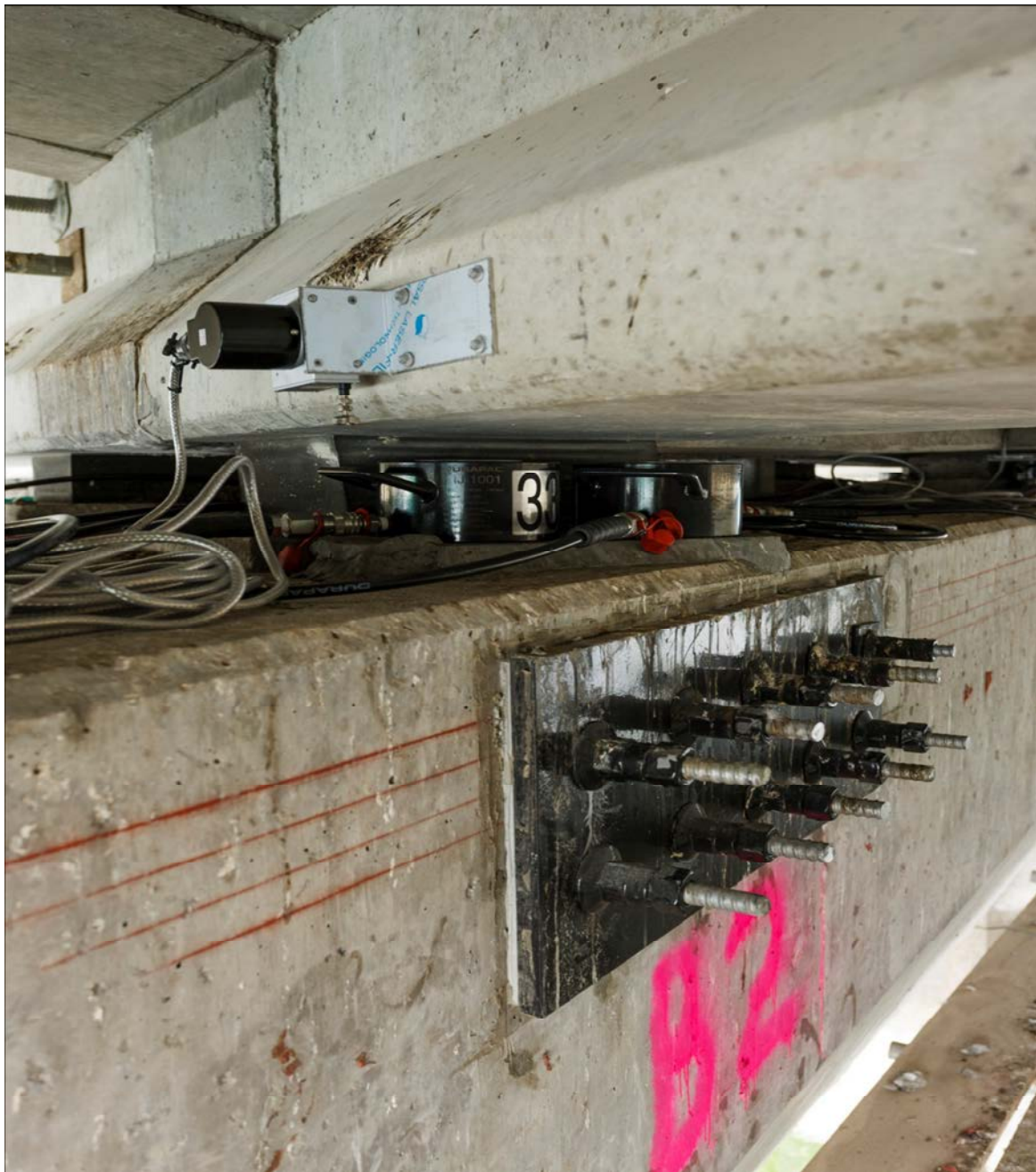
Figure 15: Low Profile Cylinders and Stroke Encoder on Pier
